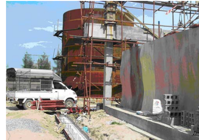
Demineral water plant
