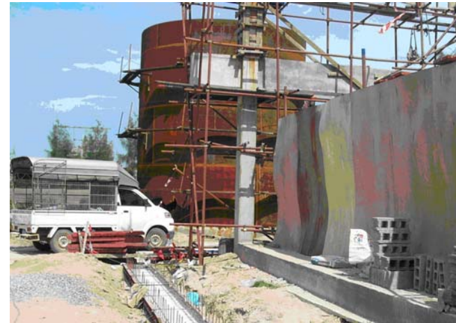
Demineral water plant
